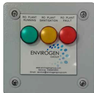
Remote wall-mounted alarm indicator
